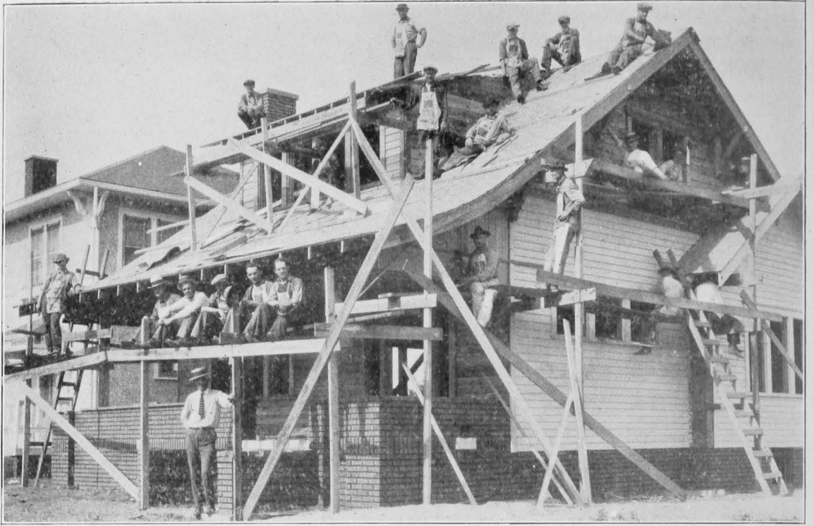
Practical work in carpentry showing the results at end of four weeks of work.
